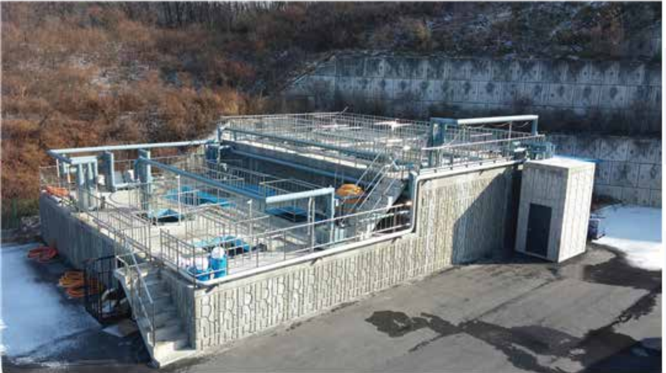
DMF (Dimethylformamide) Wastewater treatment plant
